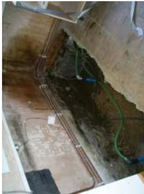
Photograph 4: Two SVE points installed in the soils within the kitchen of No.10.
