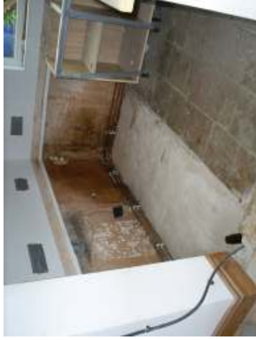
Photograph 6: View of the SVE system installed into the wall within property No. 10.
