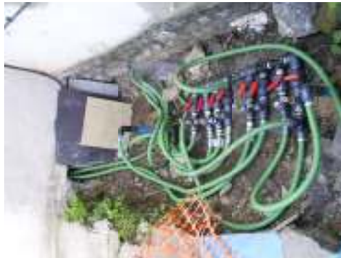
Photograph 1: The excavated floor in the kitchen of No. 10 to remove impacted soils to foundation level.
