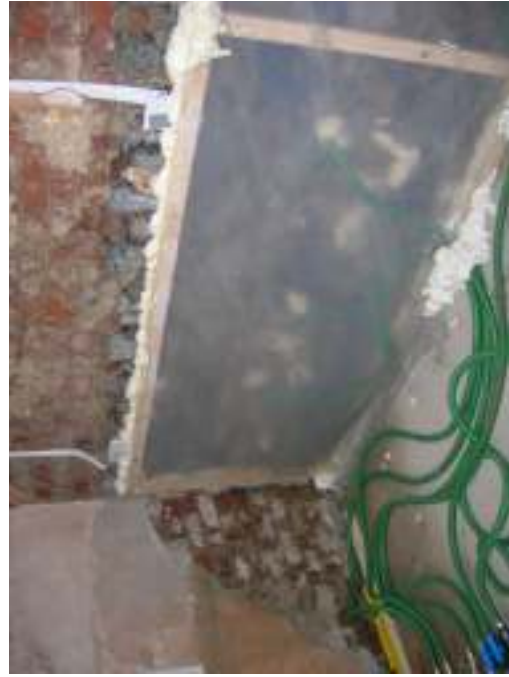
Photograph 5: View of the SVE points installed into the soils within the kitchen of No. 12.
